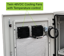
48V DC fans to keep batteries cooler.
