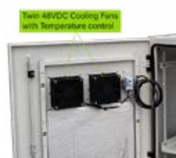
48V DC fans to keep batteries cooler.
