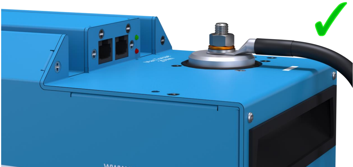
Figure 17 - Good connection of power cable
