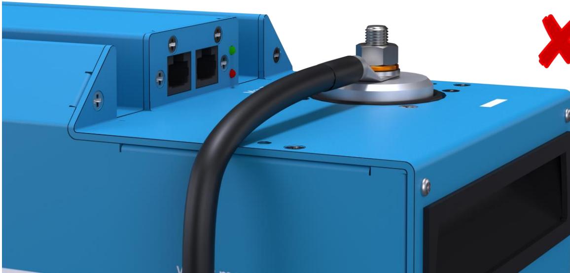
Figure 16 - Wrong connection of power cable
