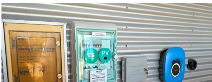
EV charging provision
