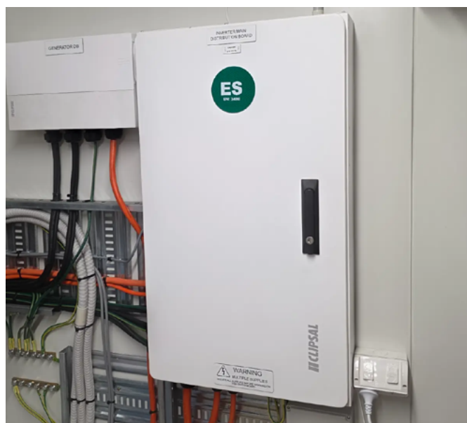
Distribution and control equipment
